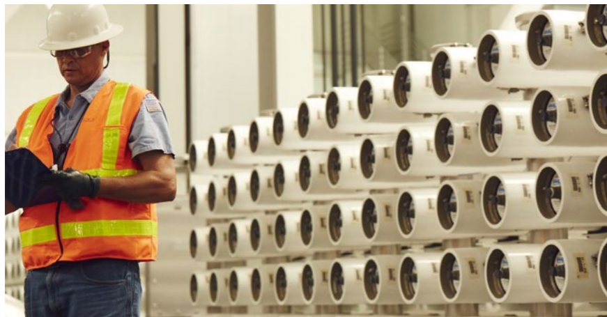
Image of the facilities of the Groundwater Replenishment System project. Photograph taken from the Orange County Water District website.
